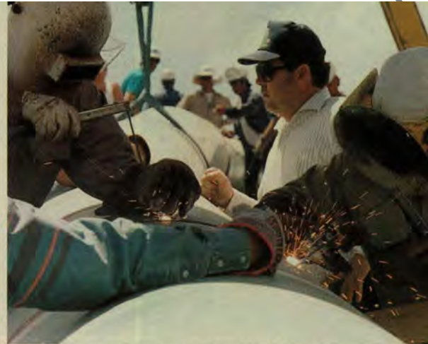
Local 342 Pipeline Representative Steve Mikich (center) inspects some of the work on the central California section of the pipeline.
