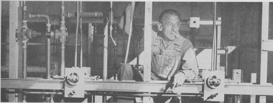
BROTHER JOHN V. KLEIN of Local 444 worked on the construction from its beginning to its completion. He firmly believes once he starts working on a job, he should remain until its is finished.
