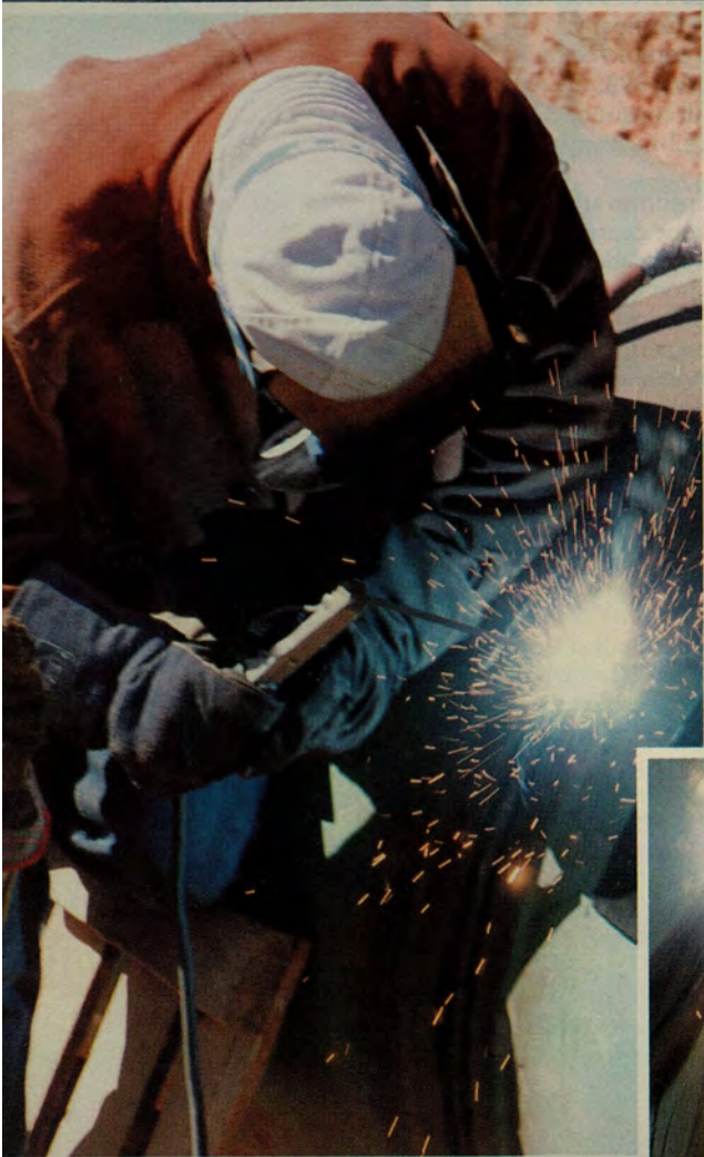
Local 342 Welder Don Gianini working on the San Joaquin Valley portion of the pipeline.
