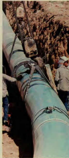
The tie-in crew at work after the pipe is lowered into the ditch.
