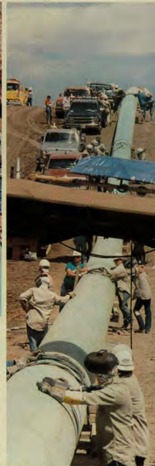
The hot pass crew (front) is followed by the hot filler crew and their rigs (back), in a carefully coordinated and timed procedure.
