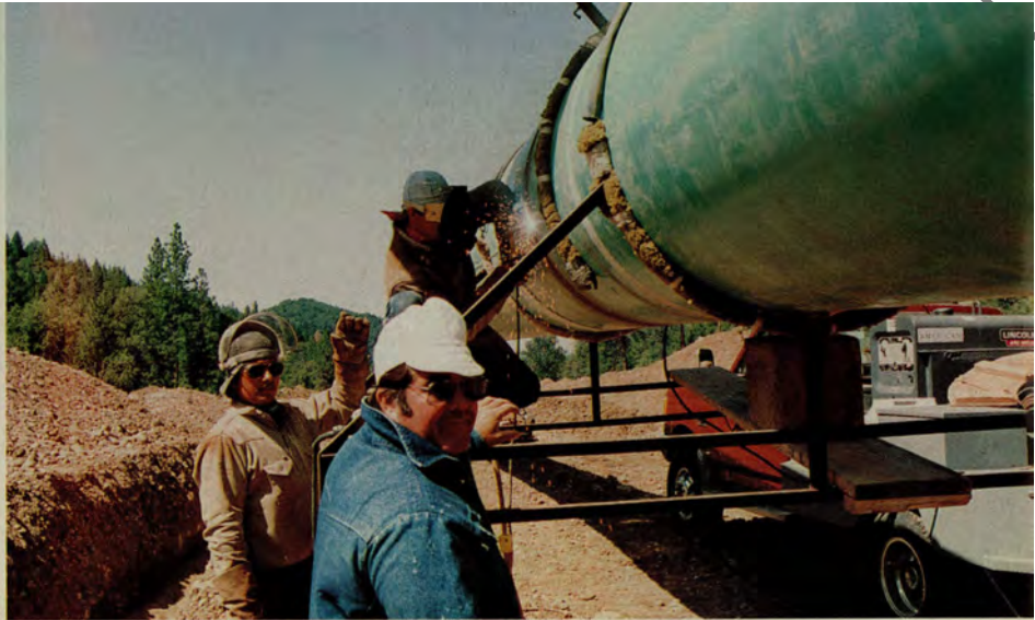
Local 342 member Merle Sandy, the job steward for H.C. Price, meets with welders working on a portion of the pipeline in Northern California.
