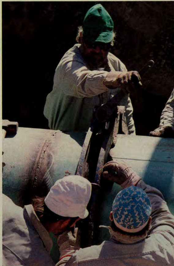
Pipeline welders at work performing a section of road bore on the San Joaquin Valley pipeline.
